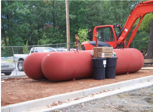
Underground LP gas tanks
