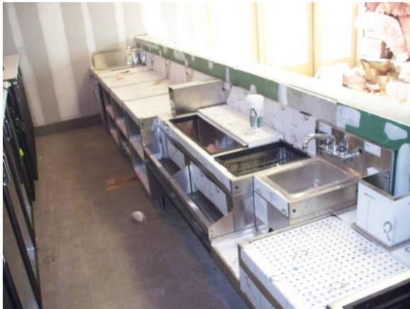
Kitchen equipment at grill
