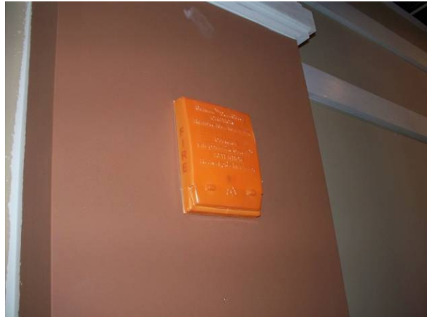
Fire alarm device with dust protection
